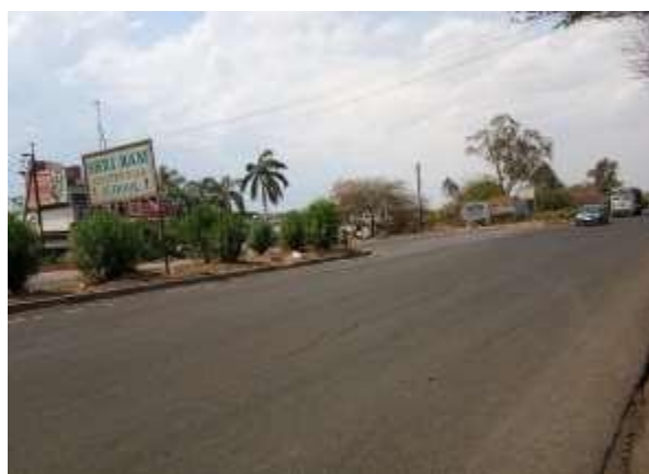
Fig 8. Condition of road on Baroli Toll Plaza to Shri Vaishnav Vidhyapeeth Vishwavidhyalaya U-Turn.
