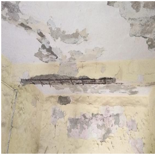
Fig.1 Exposed steel reinforcement in beam
