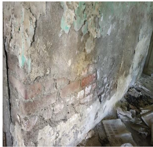
Fig.2 Dampness in wall
