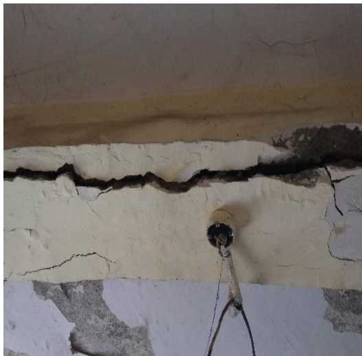
Fig.3 Crack in beam
