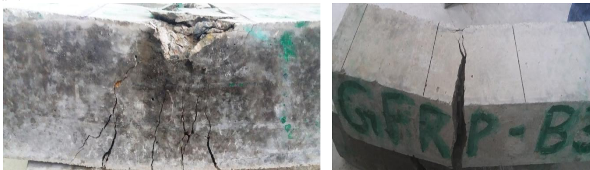
Figure 4 Crack Pattern in Steel and GFRP bars reinforced Beams
