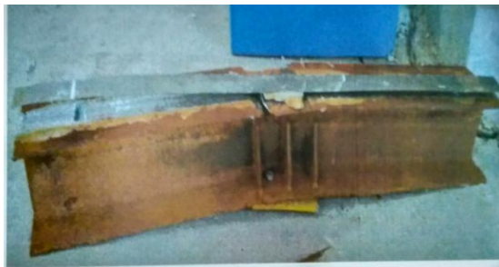
Fig. 12 complete steel and adhesive interface de-bonding
