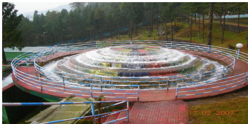
Figure-2- Aeration unit
