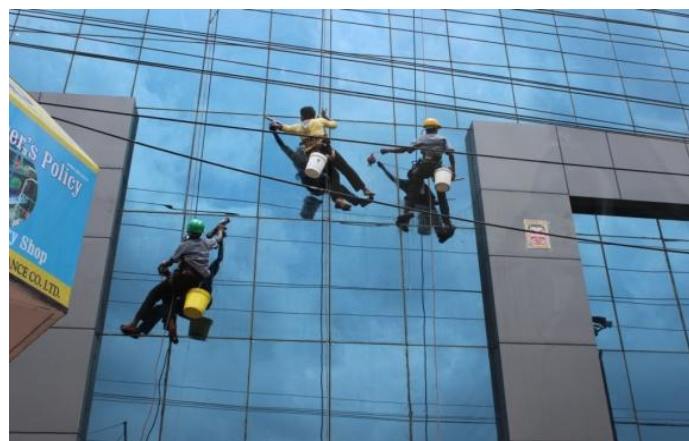
Fig:-1 Suspended box for cleaning glass wall
