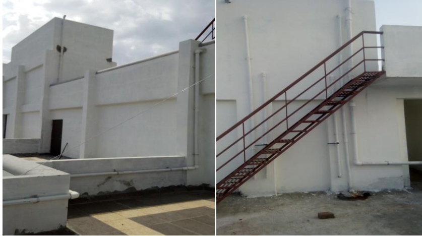
Fig.6 Over Head Water Tank (Actual)
