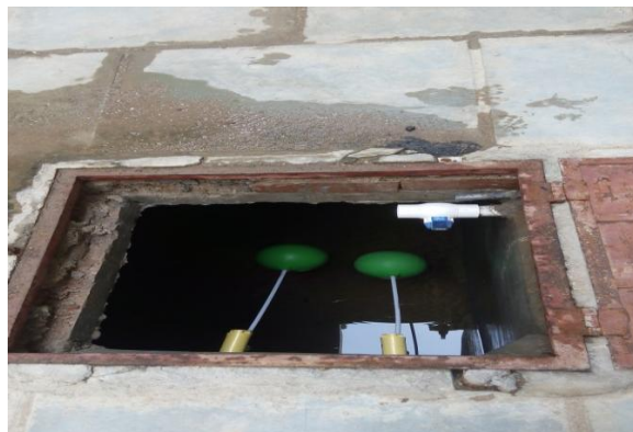
Fig.7. Underground Tank with ball valves
