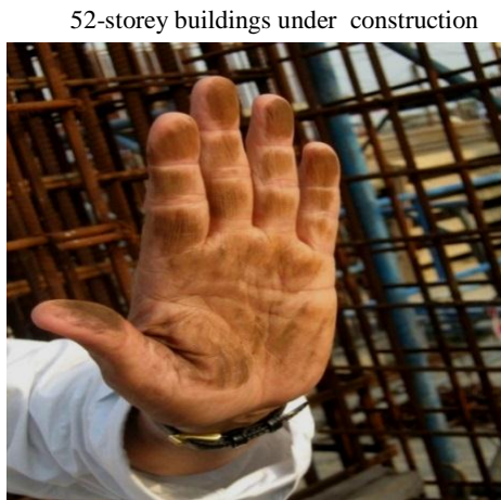
(e) : Ribbed TMT bars coated with products of corrosion even before concreting (designer one of the top designers in the world • contractor one of India's best • rebars manufactured by one of India's best known manufacturers • there was quality control by a team of engineers from a university)
