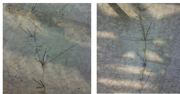
(f) : Through-the-thickness cracks in reinforced (with ribbed TMT bars in the figure above) concrete shear walls for tall buildings in Kolkata even before a floor was completed (project has top designer, proof design consultant, leading rebar maker, top contractor and quality monitoring agent) in 2011
