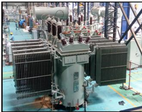
Fig. 1. Temperature rise test setup.
