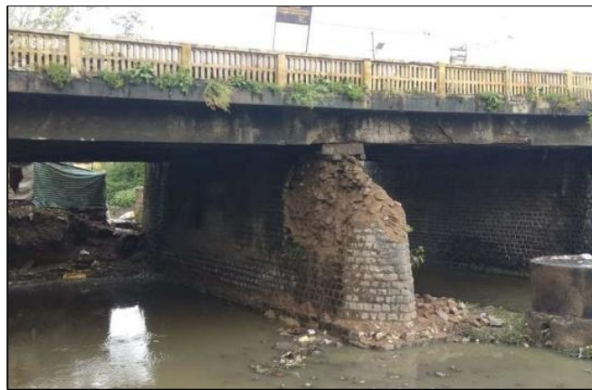
Fig.6 Bridge weakens brick by brick
