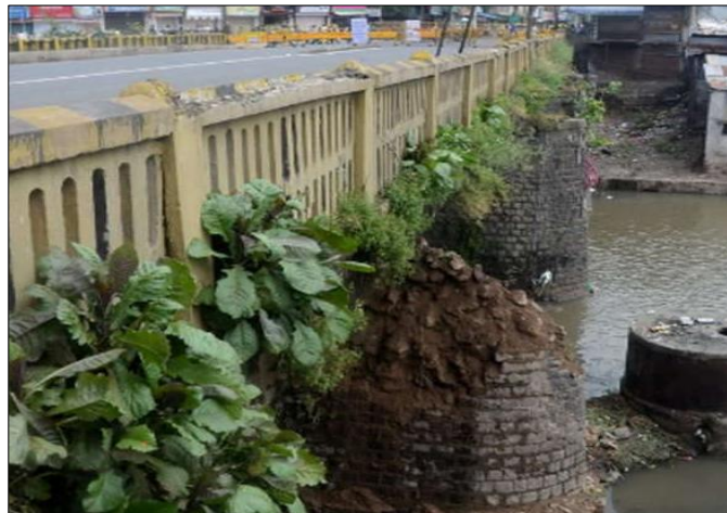
Fig. 5 Bridge damaged due to heavy rain.
