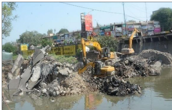
Fig.6 the 65-yr-old bridge had collapsed after the rains
