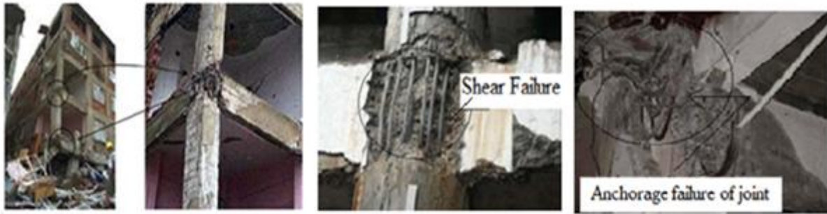
Non- Seismically detailed Beam-column joint by Shear & Anchorage failure
