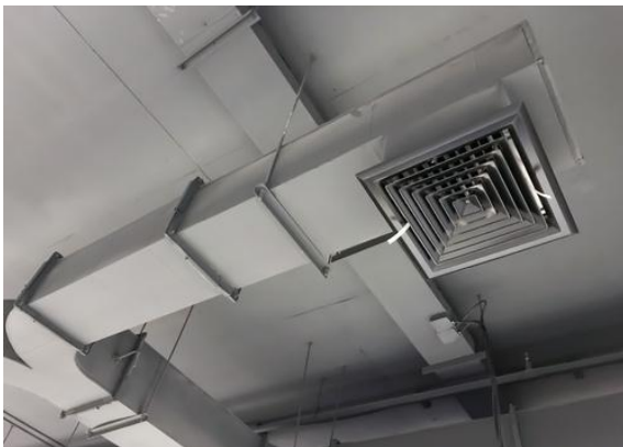
Fig 1: Commercial building HVAC duct system
