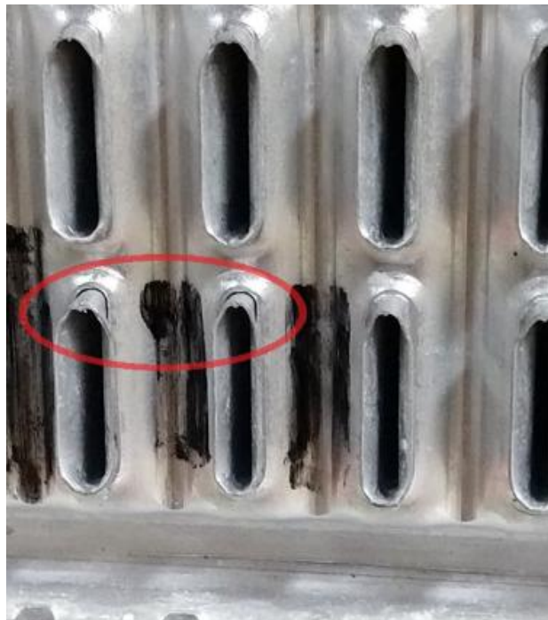
Figure 4 Header plate to tube joint leakage
