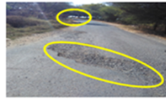
Figure 5.6: CH-1423.25m. Pot holes, no curvature markings
