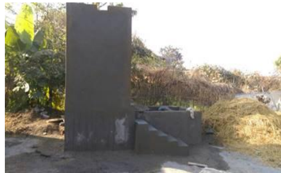
Bio-toilet under construction in Raigarh (note- it is constructed in hard rock terrain therefore entire tank is constructed above ground)
