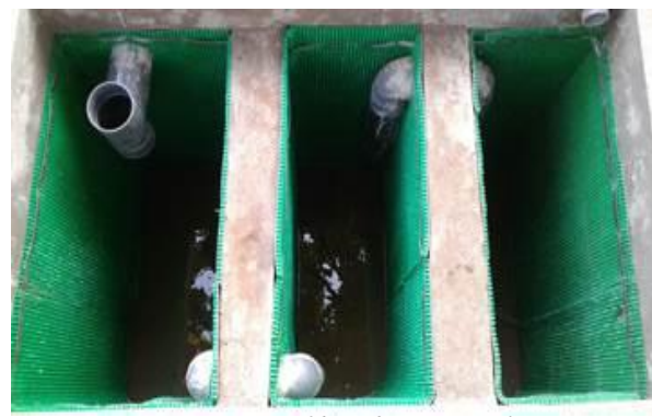
Innner view of bio-digester tank
