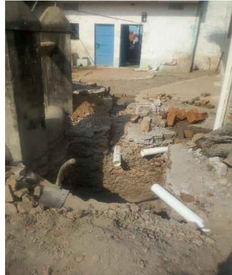
After Filter Chamber pipes coming to recharge pit
