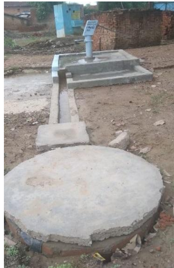
Recharge pit nearby India Mark II handpump
