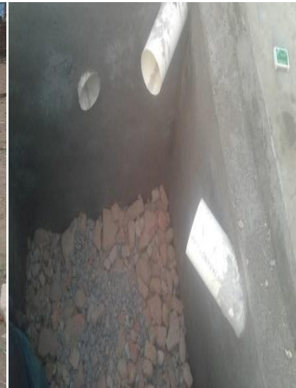
Chamber pipes connected to Recharge pit
