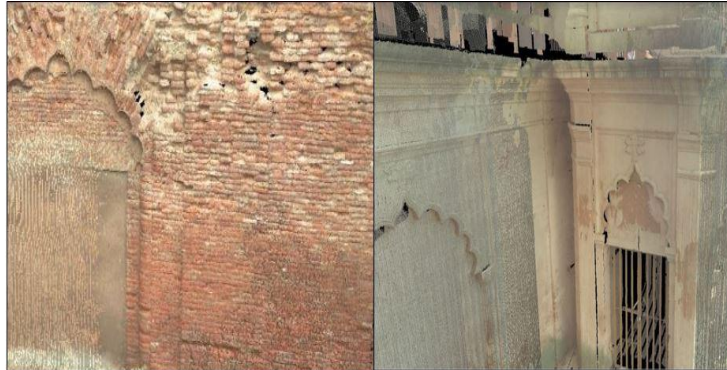
Figure 7 TLS data showing the deterioration in the both structure.
