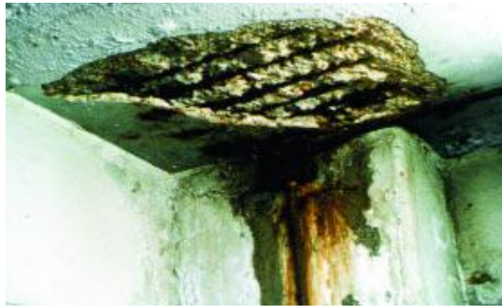
Fig. 1. Corrosion of reinforcing steel is the most common cause of concrete deterioration. (46080)
