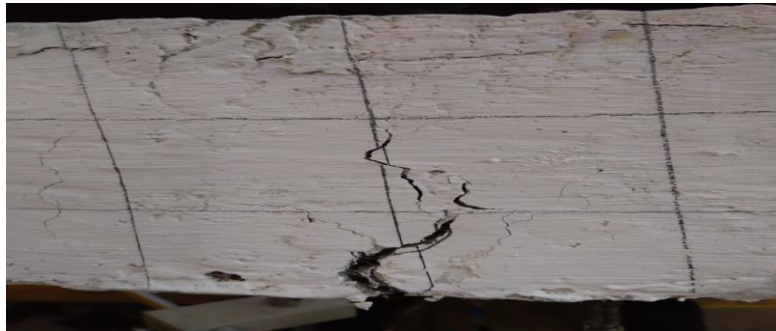
Figure: 5 Failure pattern of the beams
