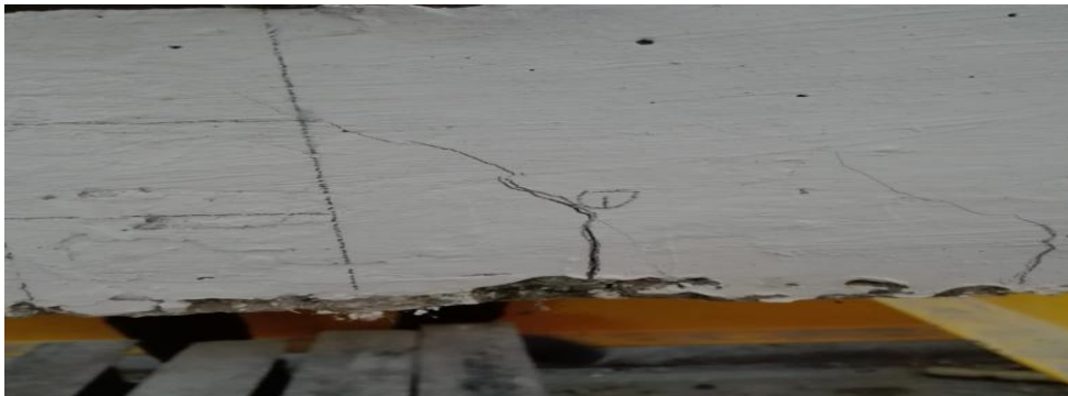
Figure: 6 First crack of RC beams
