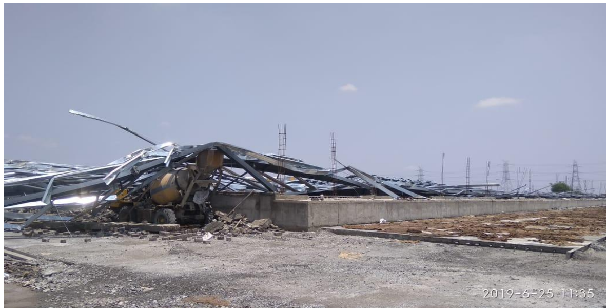
Fig. 3 Typical condition of remaining structure
