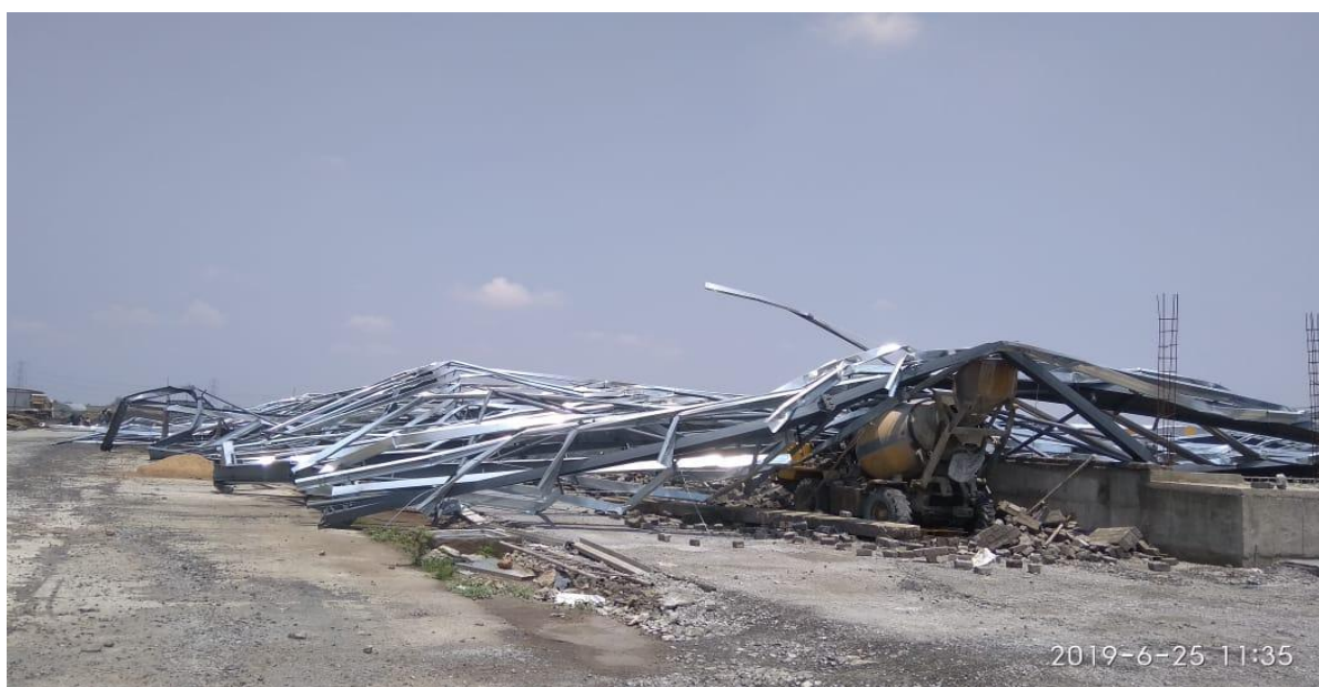
Fig. 4 Collapsed Coldstore Structure
