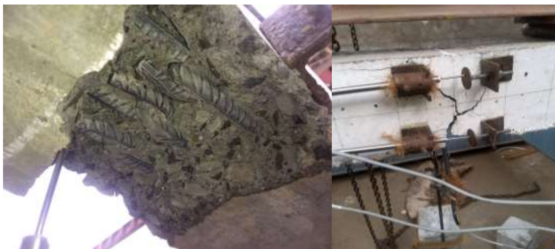
Fig 4 Cracks in beam with hook reinforcement
