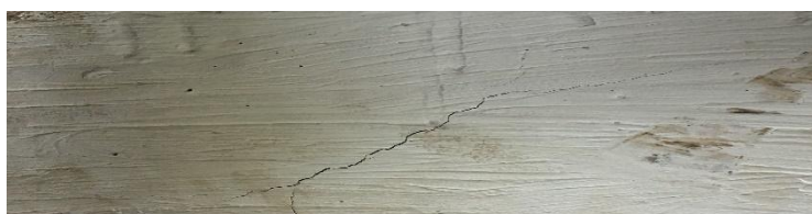
Figure 9: Crack found on RCC beam using Vertical stirrups
