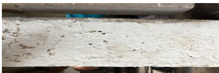
Figure 10: Crack found on RCC beam using Combination of both stirrups
