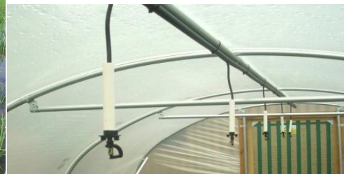
Figure 2 Overhead Irrigation Systems
