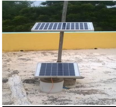
Fig.1 Vertical arrangement of solar panels at 0.75m distance
