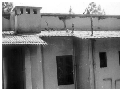
Fig. 9 Damage to wall supporting Split Level roof - ITBP campus, Mahidanda, Uttarkashi Earthquake
