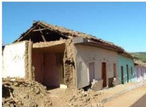
Fig. 5 Out of plane failure in Maule Earthquake.
