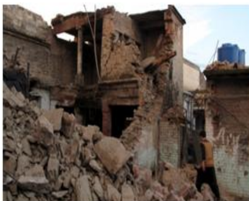
Fig.15 Partially collapsed structure in Afghanistan–Pakistan Earthquake
