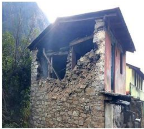
Fig.12 Out-of-plane failure in Chamoli Earthquake
