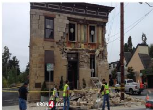
Fig.16 Out-of-plane failure in South Napa Earthquake
