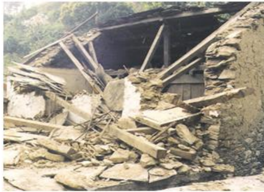
Fig.13 Partially collapsed structure in Basyurt-Karakocan (Elazig) Earthquake
