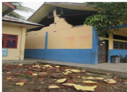
Fig.14 Collapsed masonry building in Pidie Jaya Earthquake
