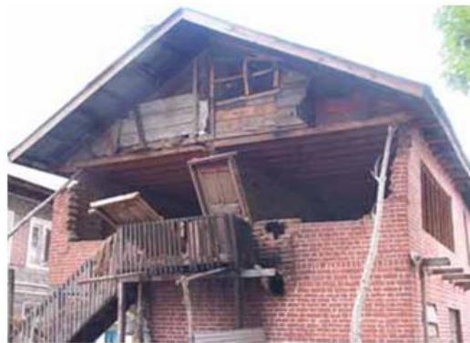
Fig.18 Out-of-plane collapse in Kashmir earthquake
