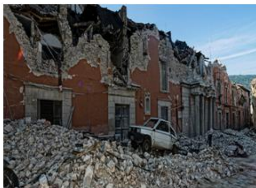
Fig.17 Out of plane failure of building in Molise Earthquake
