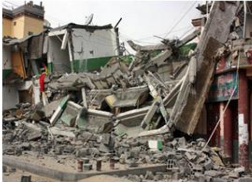
Fig.19 Fully collapsed of the structure in Lushan Earthquake
