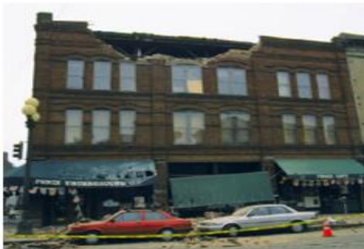
Fig.20 Brick Parapet and Wall Failure in Nisqually Earthquake
