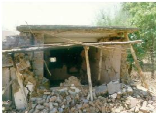
Fig. 11 Partially collapsed of the structure in Jabalpur Earthquake
