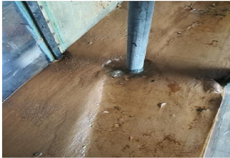
Figure 7: Scour Around Pier
